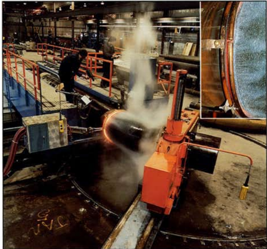
The induction bending process in operation at Indutech demonstrating the narrow heated band, controlled bending and cooling mechanisms. (Insert shows close up of inductor and quench rings.)
