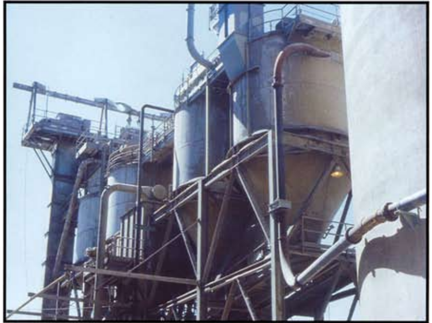
Dry Cement Handling and Storage System.
